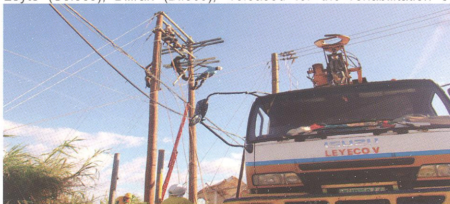
Linemen of Leyeco V begin line rehabilitation in Barangay Cogon, Ormoc City immediately following Yolanda's devastation in Nov. 2012.
